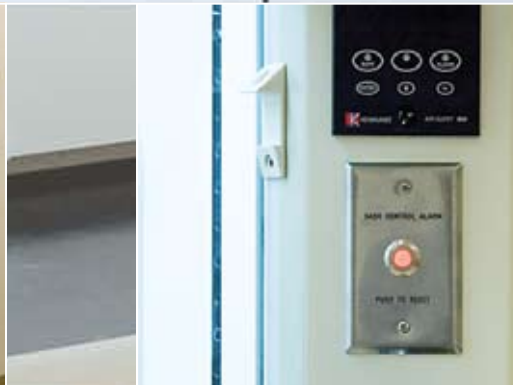
Obstruction Warning Light
